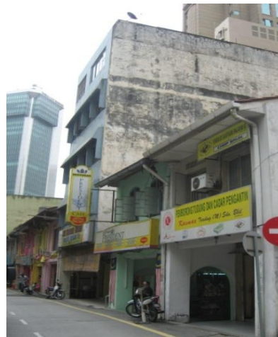
Figure 15: Using inappropriate materials such as concrete in shophouses
